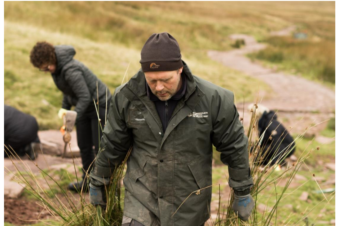
National Trust Rangers and volunteers repairing the mountain footpath at Pen Y Fan
